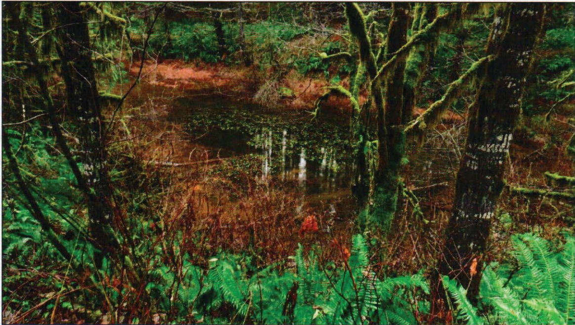
Figure 5: Stream flow impounded by undersized culvert, causing ponding, on Loveland Bay Road
