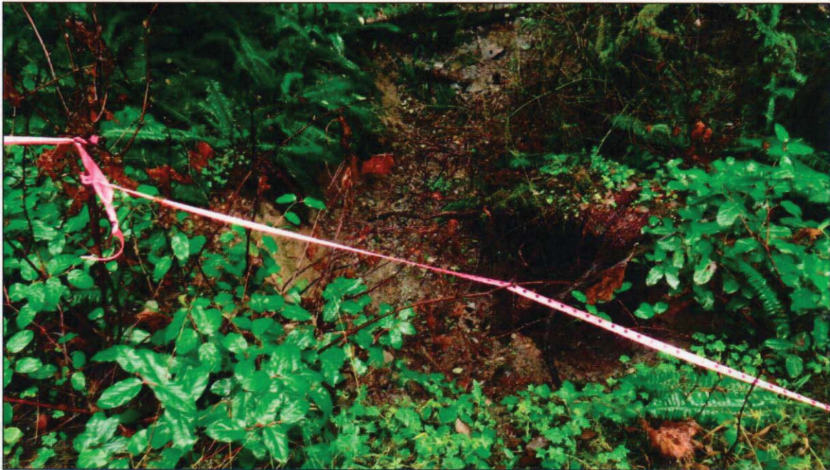
Figure 4: Thick, oversteepened road fill and slumping on Loveland Bay Road at stream crossing
